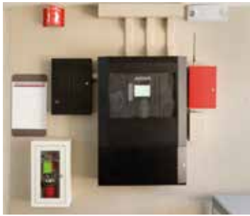
Security and fire alarm
