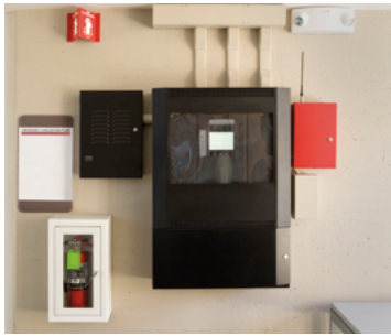
Security and fire alarm
